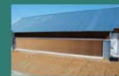
Cooling Pads & Fans
